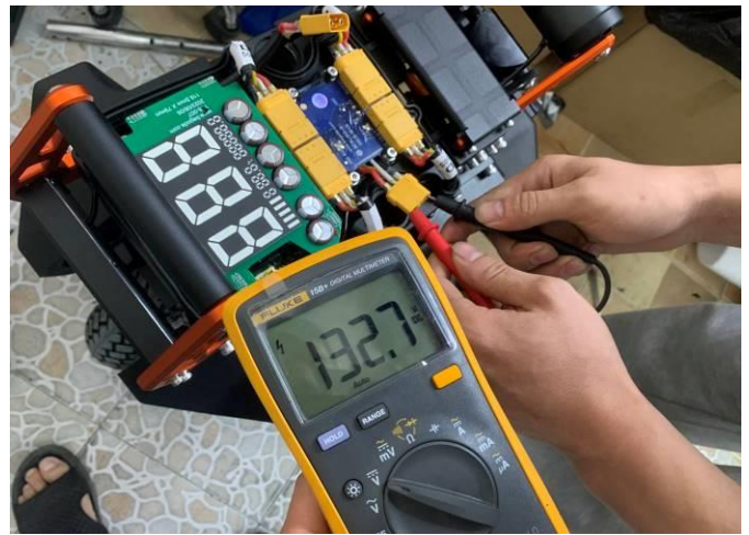
6 Battery voltage check
