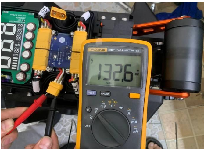
5 Battery voltage check
