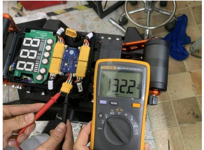
4 Battery voltage check
