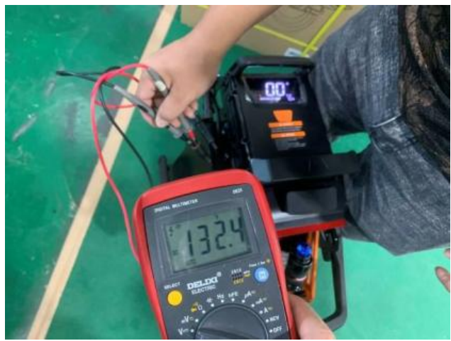
Battery voltage check
